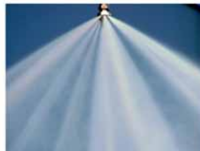
Impianto water mist
